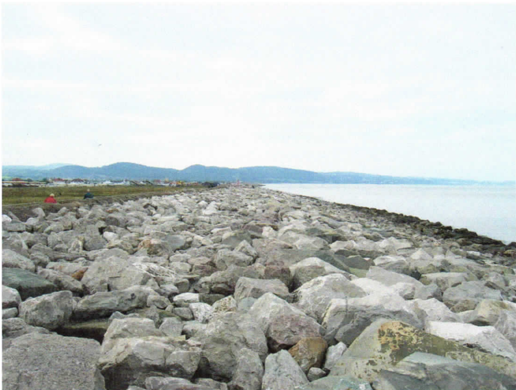
Plate 6. Seaward face of new Towyn defence (Section B)
